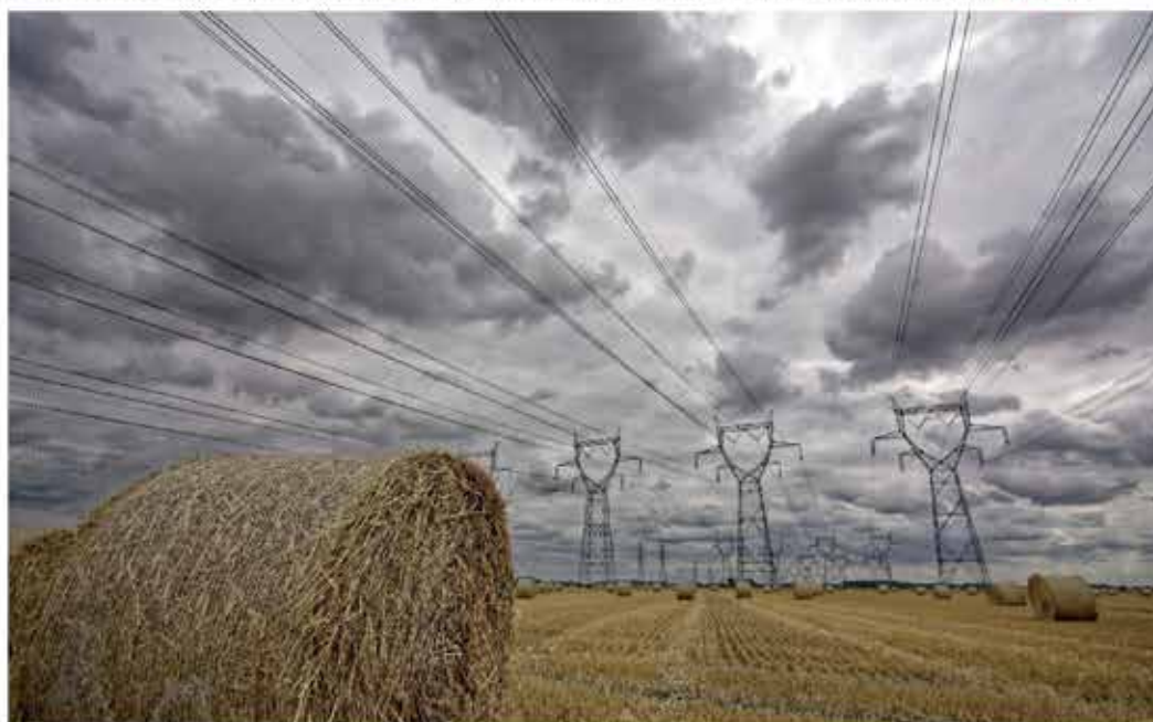
Figure 3: example of suspension towers for 400 kV overhead lines
